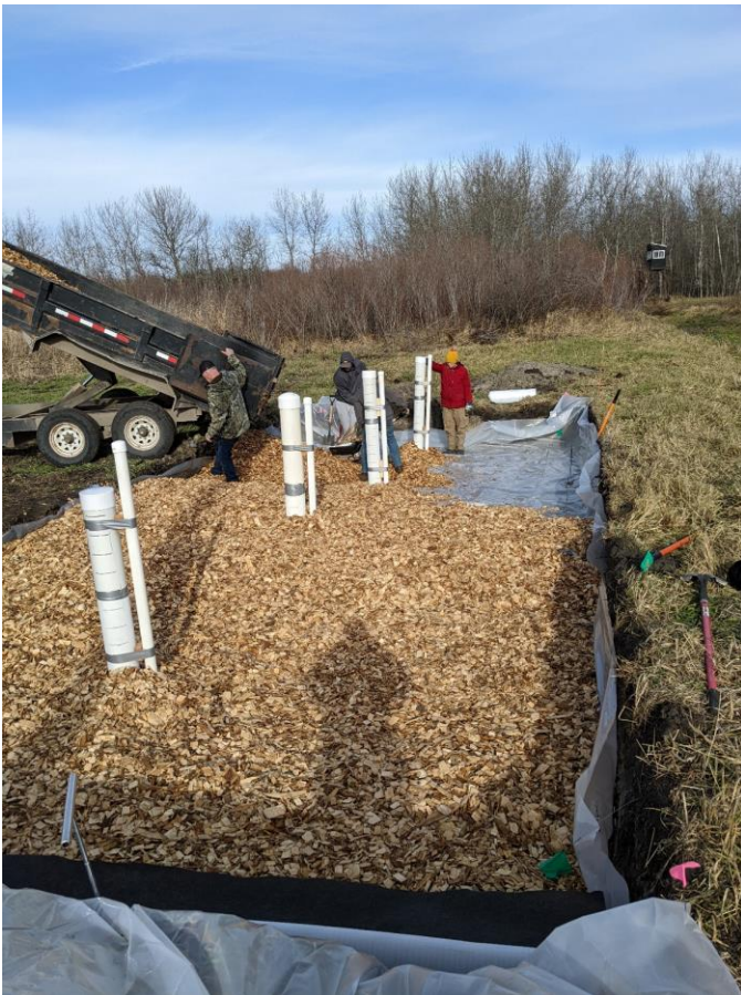
Four monitoring wells were installed in the middle of the bioreactor as it was being filled with woodchips
