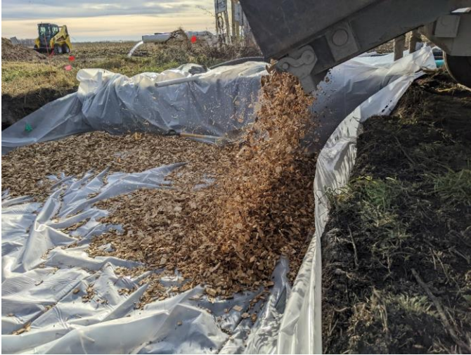
Woodchips being dumped into the lined, excavated pit during construction of the bioreactor in November 2023.
